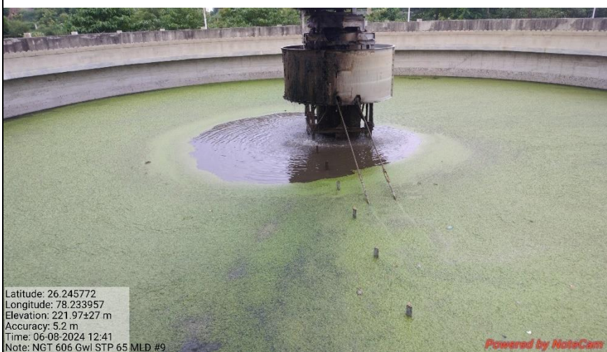
Algae present in Sludge thickner STP 65 MLD at Laltipara
