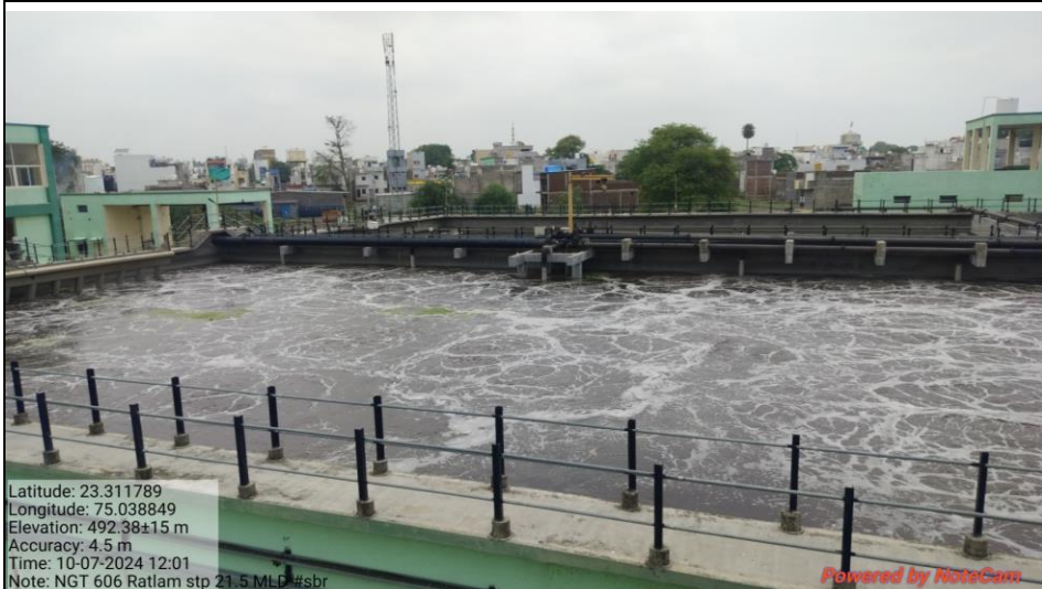
Aeration process in the SBR Basin at STP 21.5 MLD
