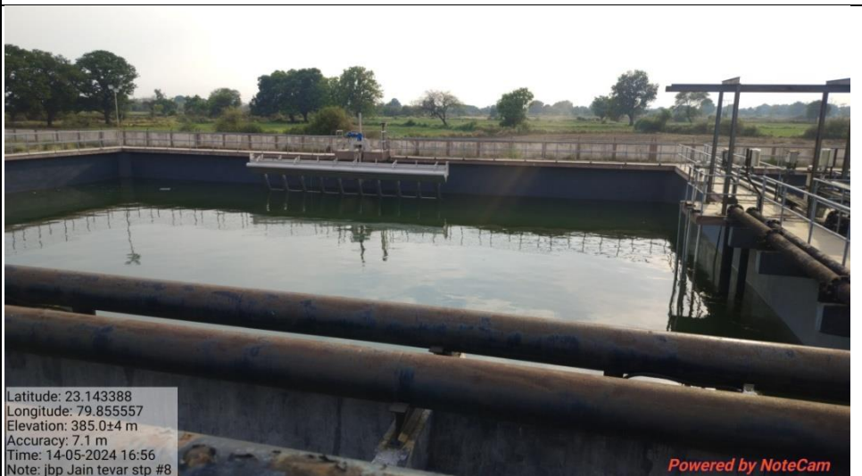
Under trail STP at Tevar (non- operational)
