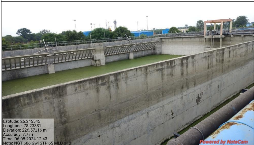
Algae present in SBR Basin STP 65 MLD at Laltipara
