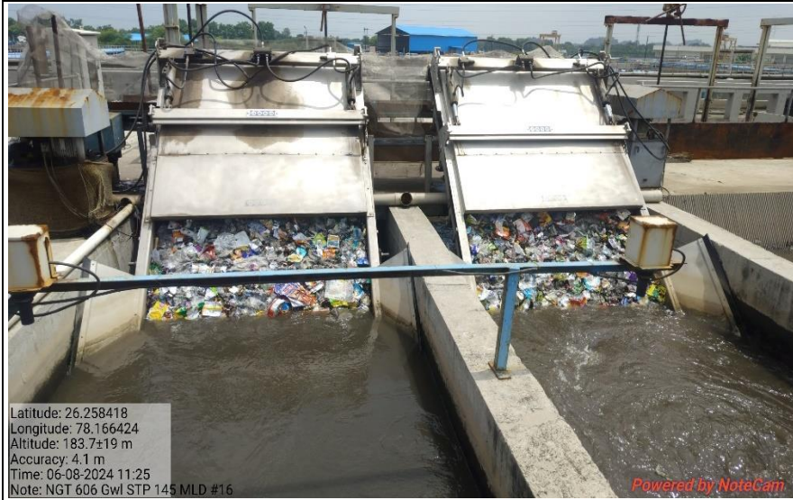
Inlet Screen STP 145 MLD at Jalalpur
