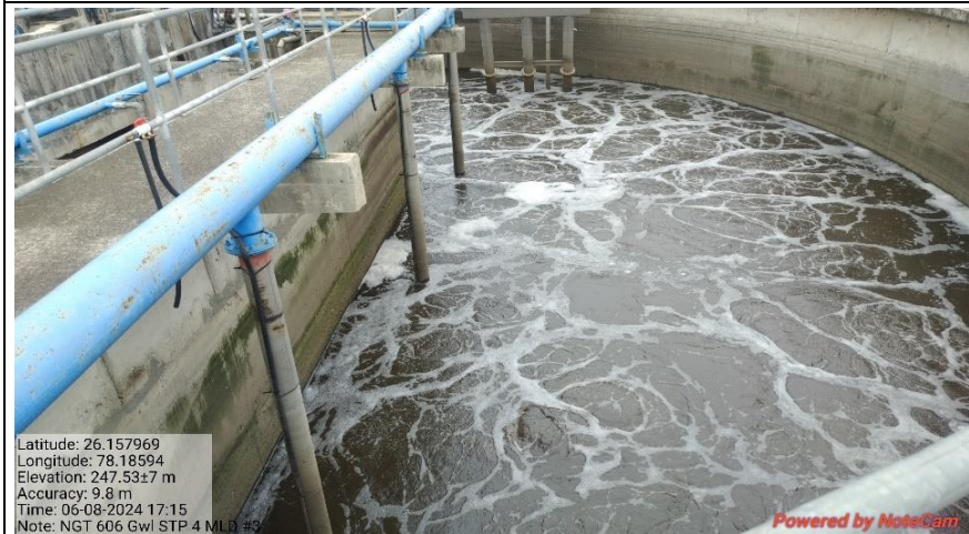
STP 4 MLD at Laliyapura
