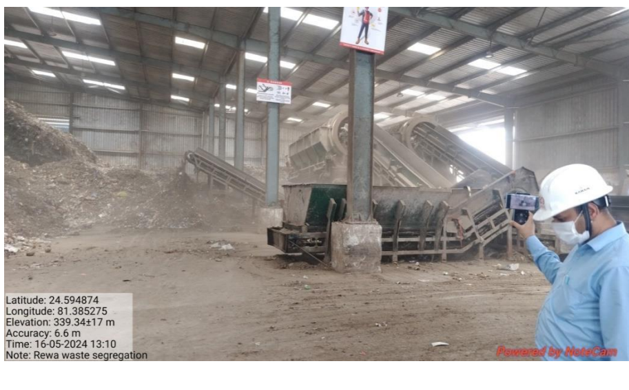
Waste Segregation at RDF Section
