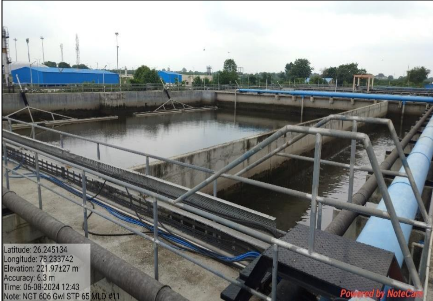
STP 65 MLD at Lalitpura
