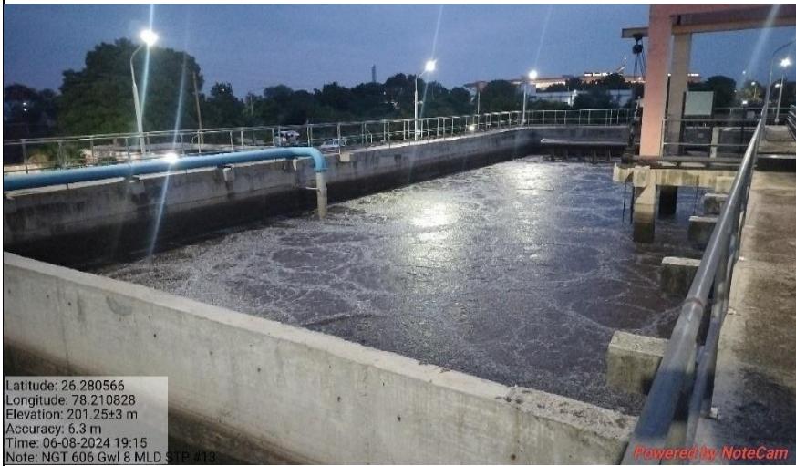
Aeration in SBR Basin STP 8 MLD
