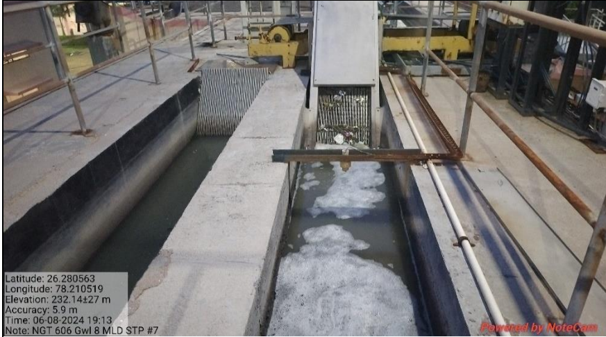
STP 8 MLD at Shatabdipuram
