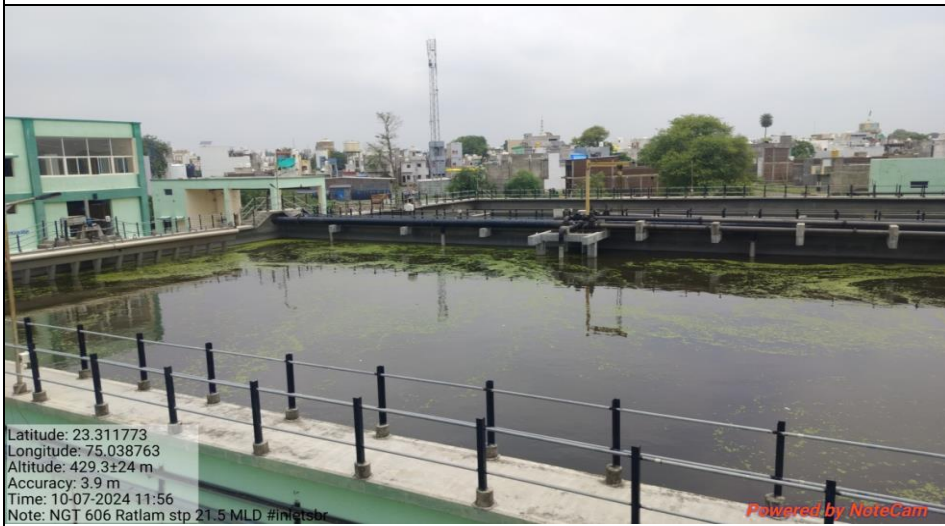
Algae in the SBR Basin at Karamdi STP 21.5 MLD
