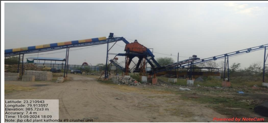
Crusher unit at C&D waste processing plant
